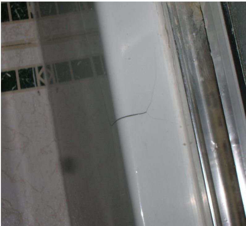
CRACK IN STEP FOR SHOWER IN 1ST HALL BATHROOM
