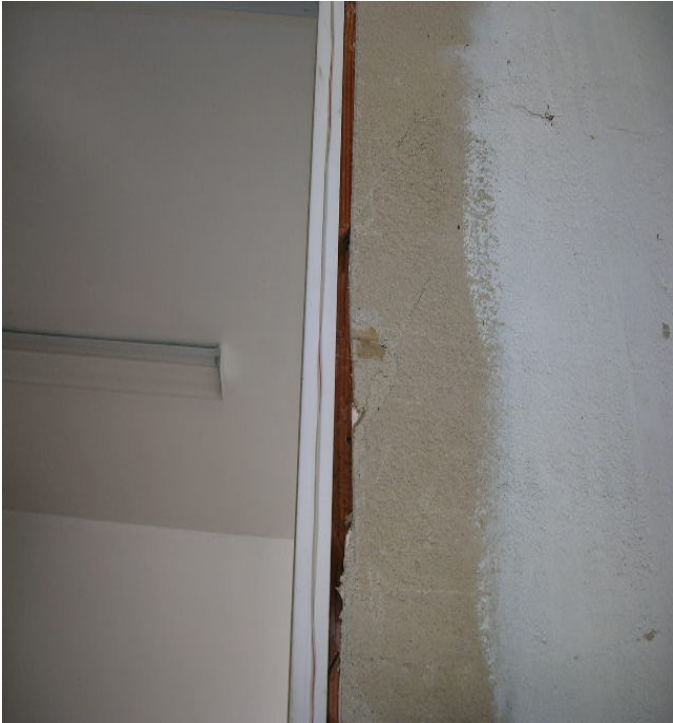
AREA AROUND DOOR NEEDS TO BE SEALED PROPERLY THIS IS A FIREWALL
