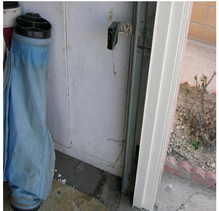
SENSORS FOR GARAGE DOOR OPENER NEED TO BE 3-4 INCHES OFF GROUND
