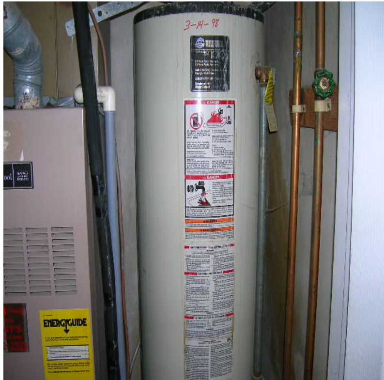
WATER HEATER NOT PROPERLY STRAPPED
