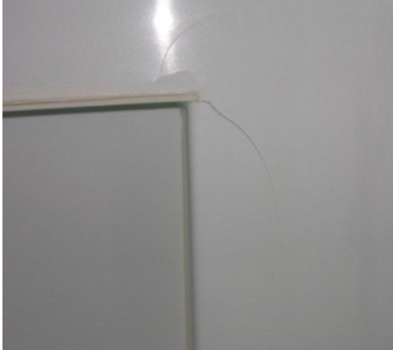
CRACK IN SHOWER WALL IN 1ST HALL BATHROOM
