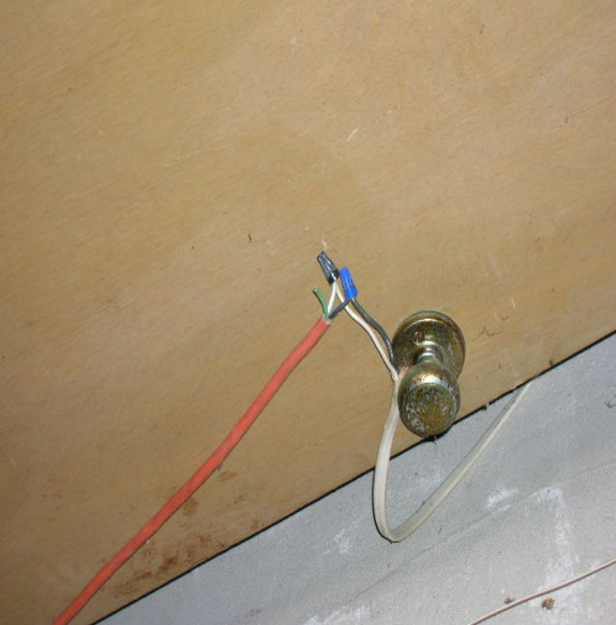
IMPROPER WIRING FOR OUTSIDE LIGHT. EXTENSION CORD TIED INTO WIRING
